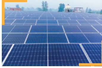
Green Earth (Pvt) Ltd., Lahore System Size: 250 kW Type of System: Grid Tied Annual CO 2 Reduction (Tonnes): 217
