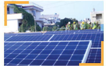
DHA Residence, Lahore System Size: 40 kW Type of System: Grid Tied Annual CO 2 Reduction (Tonnes): 35
