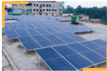
Steel Craft (Pvt) Ltd., Lahore System Size: 154 kW Type of System: Grid Tied Annual CO 2 Reduction (Tonnes): 130
